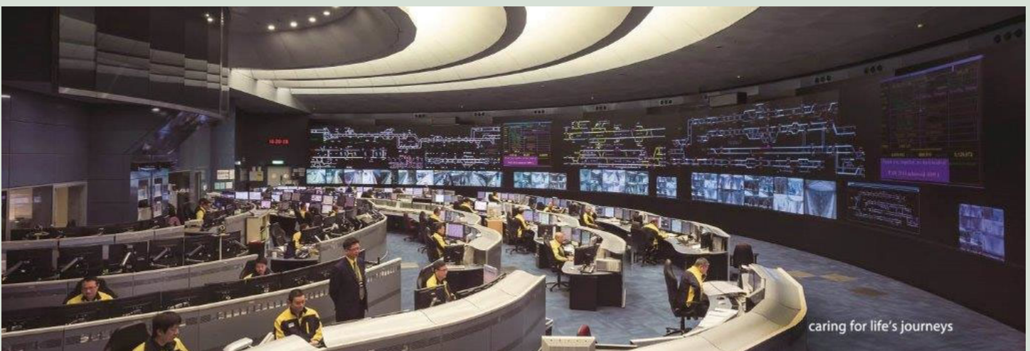
Our Operations Control Centre (“OCC”) controls the Hong Kong rail network from Tsing Yi
